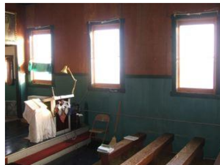
Old home-made plexi-glass windows with moisture trapped between panes
