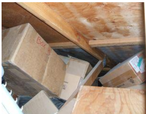
Attic space pre-Wx: Stored items compress and de-value existing insulation R-values
