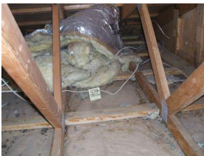
Condition of attic insulation at time of pre-weatherization assessment. Much of it was removed for some reason in the past and left uninstalled
