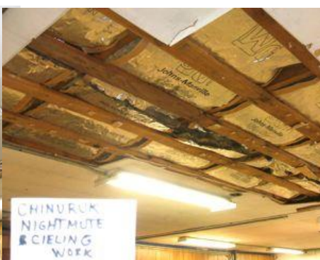
Removed ceiling tiles reveal exposed insulation and open roof area beyond
