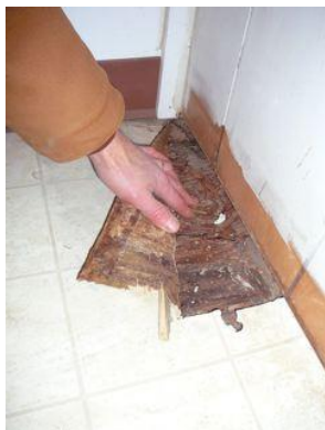
Air leakage from a dry-rotted corner. Budgets didn't allow re-building the floor, but the source of water damage had already been contained.
