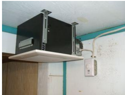
Continuous run-rated exhaust fan on timer switch installed for adding building ventilation as needed.
