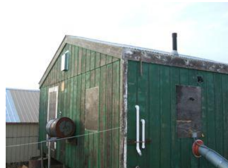
New gable-end vent with wind baffle cover
