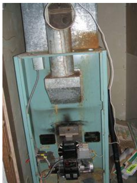
Original 40-year-old 60% efficient forced air furnace
