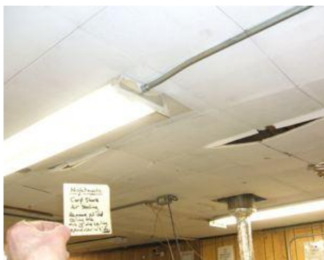
Out of place ceiling tiles leave large air leakage zones
