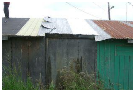
The old store was cobbled together and in very rough shape. A new roof was necessary for building viability
