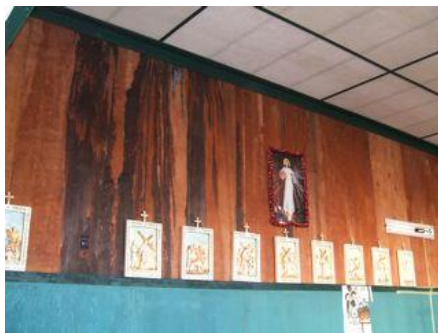
Water-damaged walls from leaking roof
