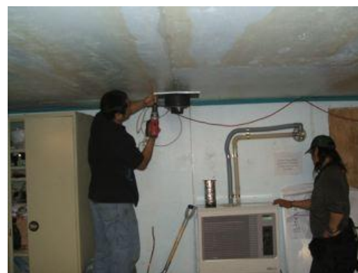
New Toyo-Stove, 84% efficient space heater installed by local technicians
