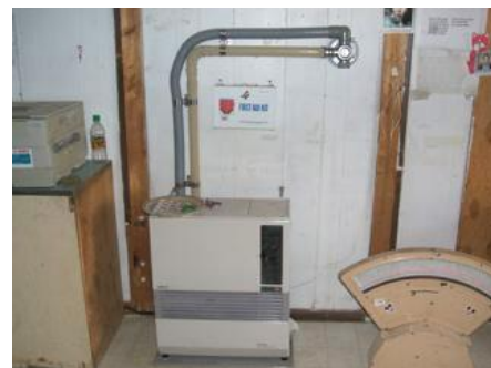
New 84% efficient space heater installed by local talent
